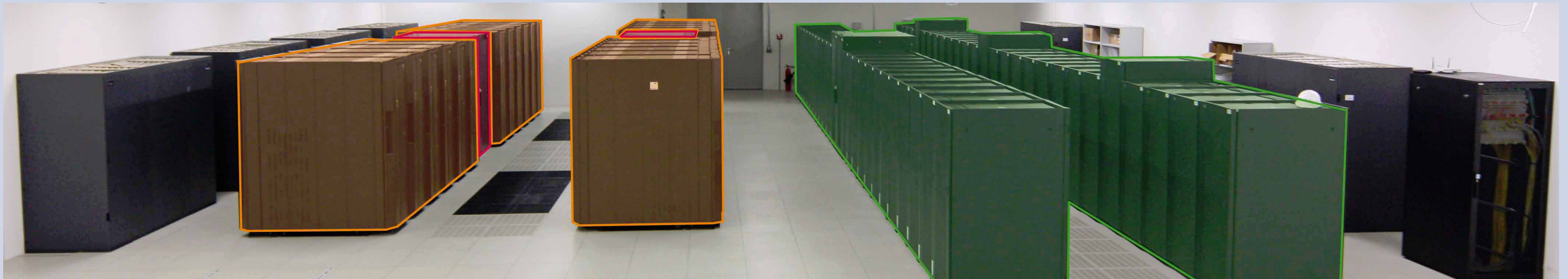
Figure 2: High performance computing system „Blizzard“ at DKRZ - compute nodes (orange), infiniband switch (red), disks (green)
