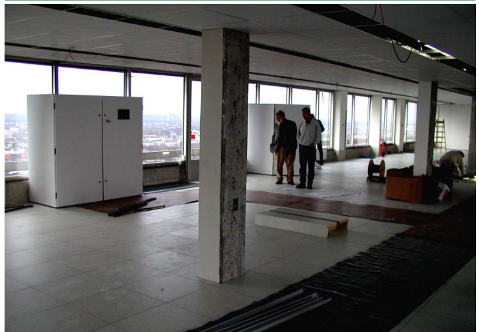
The new DKRZ computer room in the 15th floor of the Geomatikum building in Hamburg, where the SX-6 nodes will be installed in February. A whole series of photos showing the progress of the restructuring work done at our site can be found at http://www.dkrz.de/HLRE/gallery
