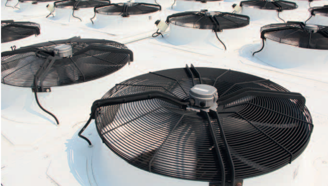
Fans are installed on the roof of DKRZ. They expel the heat produced by the computer to the outside.
